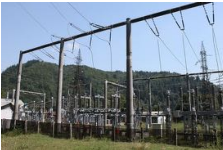
Power generation and distribution
